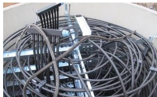
Figure 2: Empty solar ice storage unit with heat exchange pipes. Source: ZEBAU GmbH [2]
