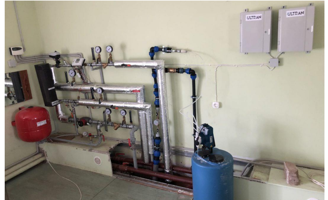
Fig. 5: Utility room LT local heating system, Photo: Sandis Kalniņš [8]
