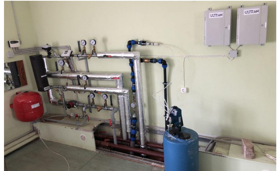
Fig. 5: Utility room LT local heating system, Photo: Sandis Kalniņš [4]
