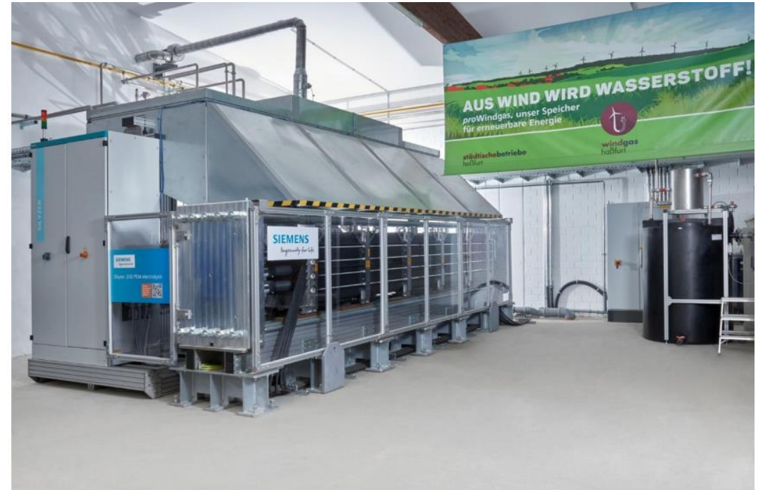
The Silyzer 200 (1.25 MW output) electrolyser from Siemens at the Stadtwerk Haßfurt is used to produce hydrogen with excess electricity from renewable energy generation plants. Image source: Stadtwerk Haßfurt GmbH
