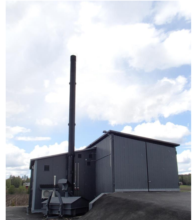
Figure 3: Heat only boiler in a sparsely populated area. Source: Thermopolis
