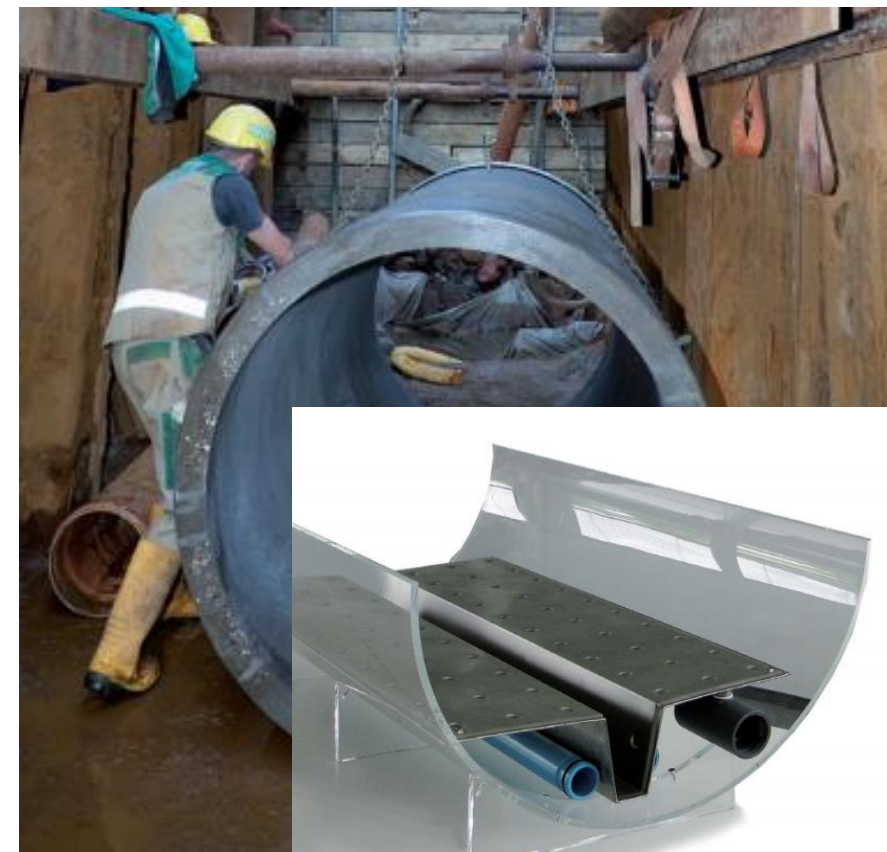
Waste water heat exchanger Source: Hamburg Wasser [9]
